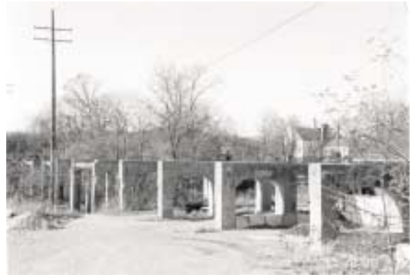
These bridge supports once carried inter-urban trains over Cahoon Creek. They could be reused to develop a walking or biking trail, which would connect the two sides of Cahoon Park and offer view of Cahoon Creek.
